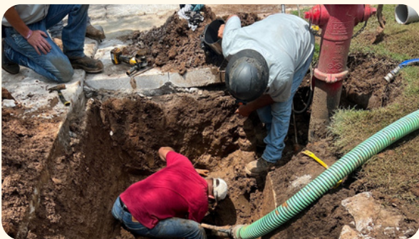
Mike Zedeker, Mike Coffman, Justin Henry, and Joe Northcutt worked during the lunch hour to make the repair.
