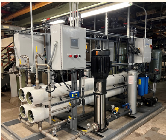
Pictured: RO Unit 1
