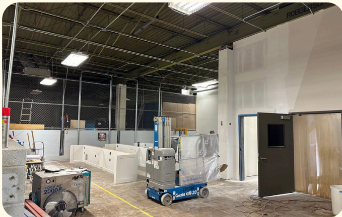
Maintenance Services - 705 Computer Lab
