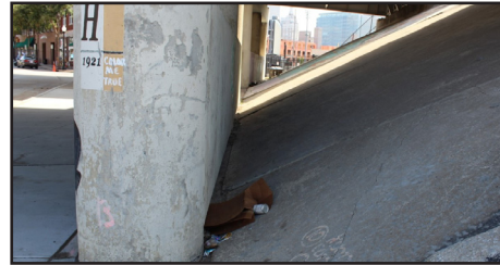
Figure 8: Photo taken on the project site of trash tucked behind the column supporting I-244.
