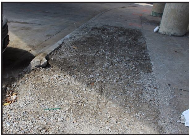
Figure 9: Photo taken on the project site in August of 2020, traveling north on the eastern side of Greenwood Avenue, under I-244.
