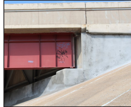
Figure 4: Photo taken on the project site of illegal tagging on the surface of the highway beam.
