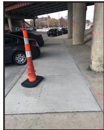
Figure 10: Photo taken on the project site in October of 2020. Photo displaying the repaired sidewalk on the eastern side of Greenwood Avenue.
