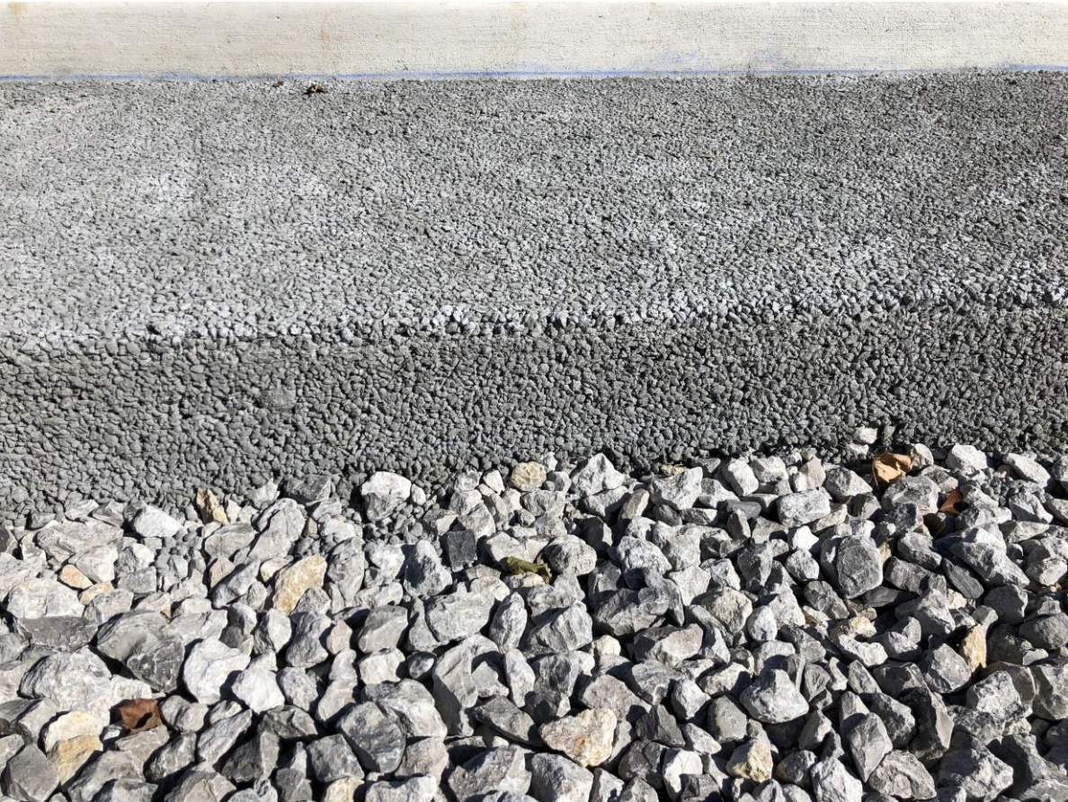
Note. Photo of pervious concrete being installed at the Claremore Baptist Church. From Clayton Harris
