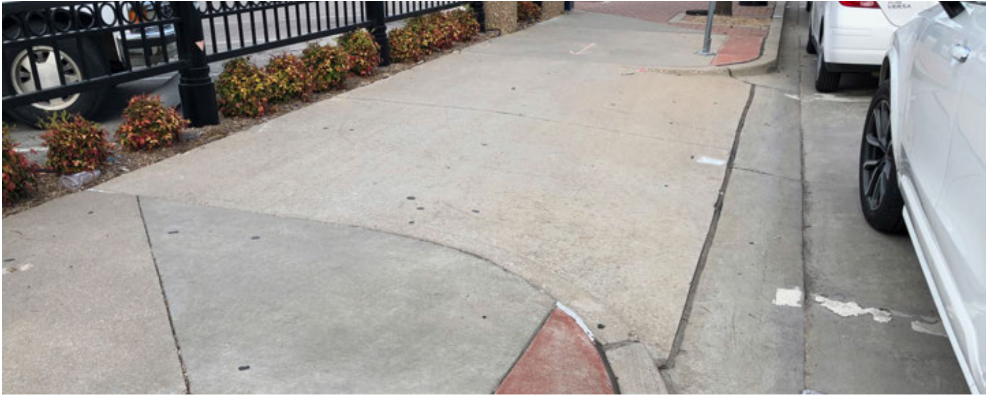
Abandoned driveways often confuse people considering parking in front of them, and create unnecessary trip and fall hazards for people using the sidewalk.
