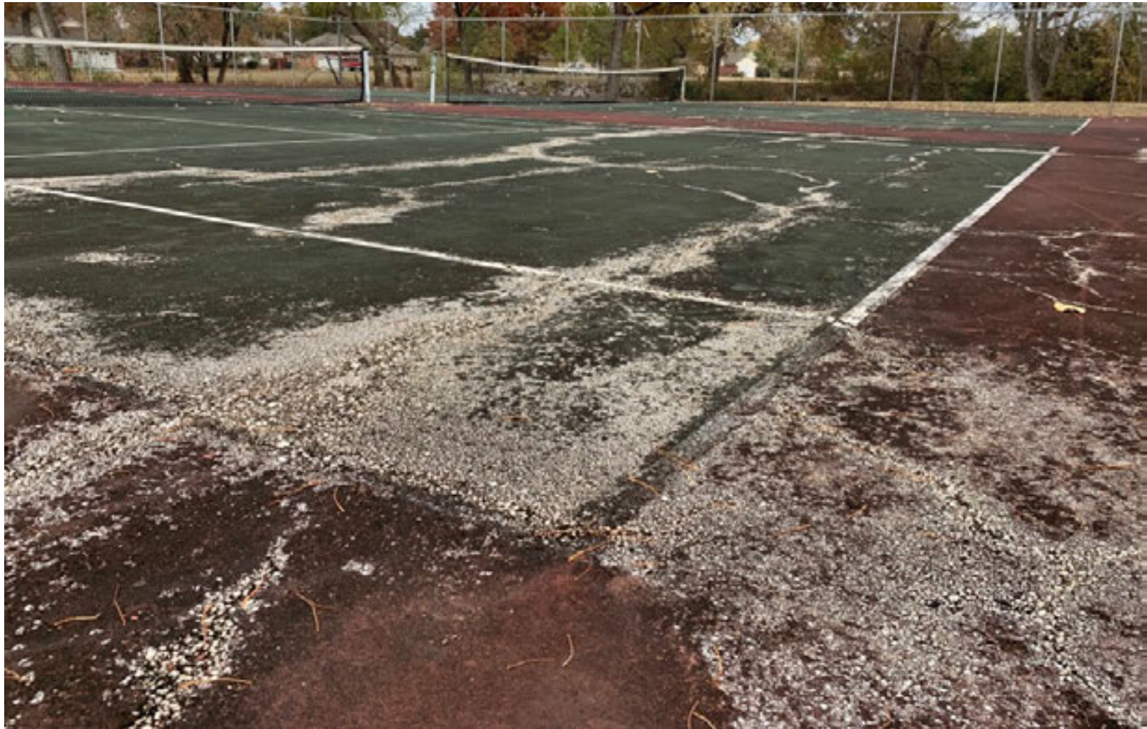
Figure 10: The tennis court surface is deteriorating, creating a poor aesthetic that can become dangerous with high activity.
