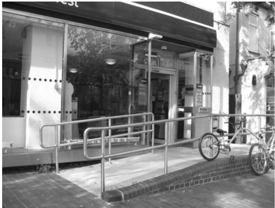
Ideally, even slight changes in level should have both a ramp and steps.
