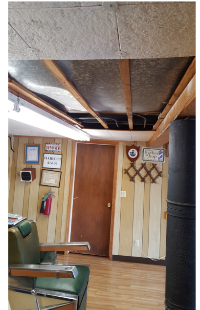
Damage to Sander's Barber Shop in Broken Arrow after the Pawnee Earthquake on September 3, 2016 illustrates the need for resilient design
