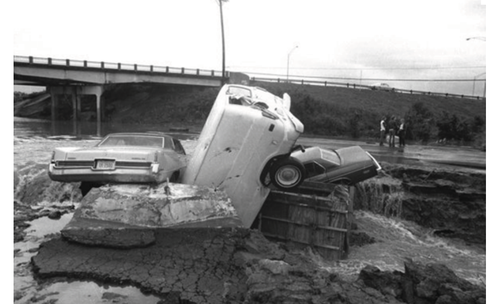
Road Damage - 1984 Memorial Day Flood http://www.tulsaworld.com/news/article.aspx?subjectid=11&articleid=20090524_11_A13_Thepow525438
