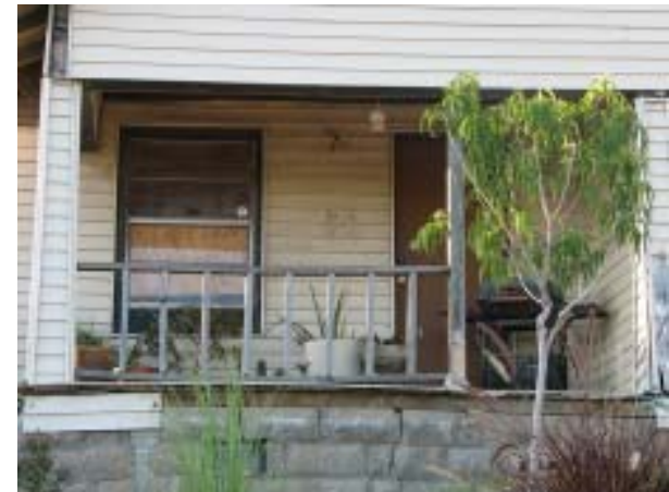
This decaying front porch is typical of conditions in the reconstruction and rebuild focus area
