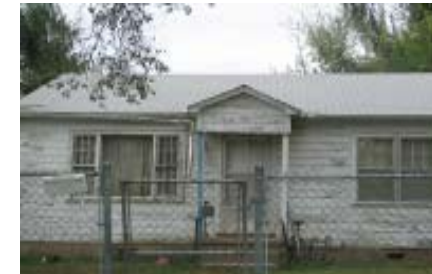
Typical North Tulsa home in decay
