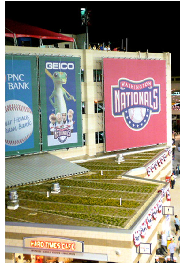
Extensive green roof on the concession stand at the Washington Nationals baseball stadium. Photo: www.greenroofs.com
