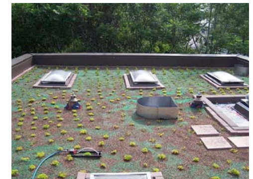
Research green roof installation during the establishment phase at the Toronto Zoo. Photo credit: http://www.toronto.ca/greenroofs/incentive_applicants07
