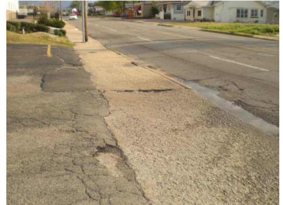
(Above) A sidewalk on the east side of Peoria Avenue shows the condition in which one finds many of the sidewalks in the Forest Orchard neighborhood. This sidewalk would be difficult to access by wheelchair as its many cracks and bumps makes it difficult for any pedestrian to use.
