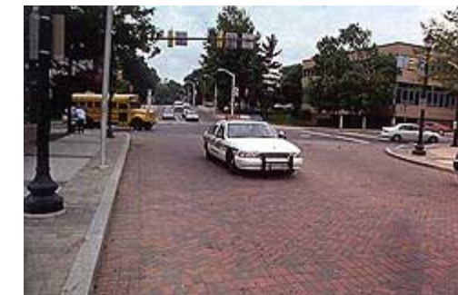
Montgomery County, MD - This textured pavement consists of evenly-placed brick, arranged in both a grid pattern and a diagonal pattern. The result is a smoother ride, less noise, and less of an effect on speeds.
